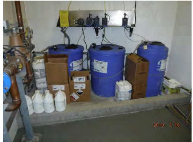
Photo 20: View of water treatment chemicals.
