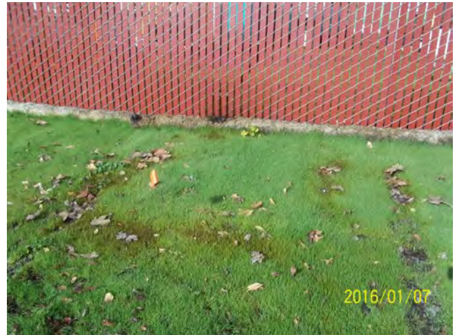
Photo 16: View of distressed vegetation associated with Photo 15 (other side of the fence).
