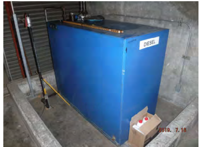
Photo 22: View of a 500-gallon diesel AST associated with an onsite generator.
