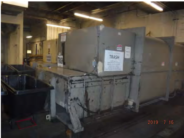
Photo 17: View of a hydraulic trash compactor.
