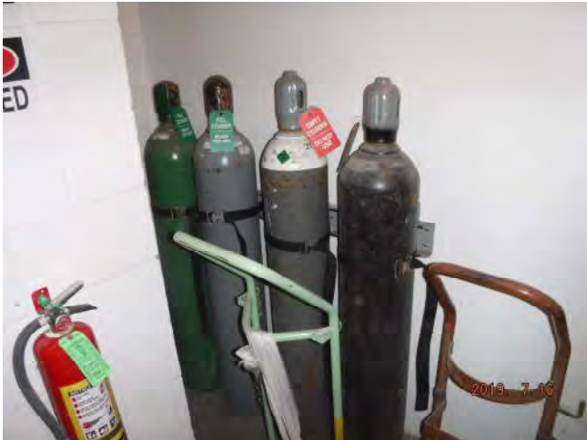
Photo 15: View of compressed gas cylinders.
