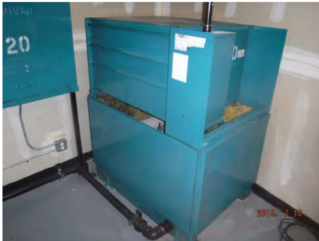
Photo 21: View of the hydraulic elevator equipment.
