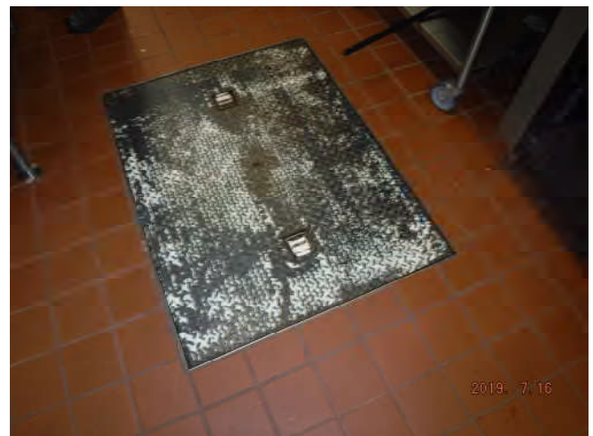
Photo 24: View of a grease trap in the cafeteria kitchen.
